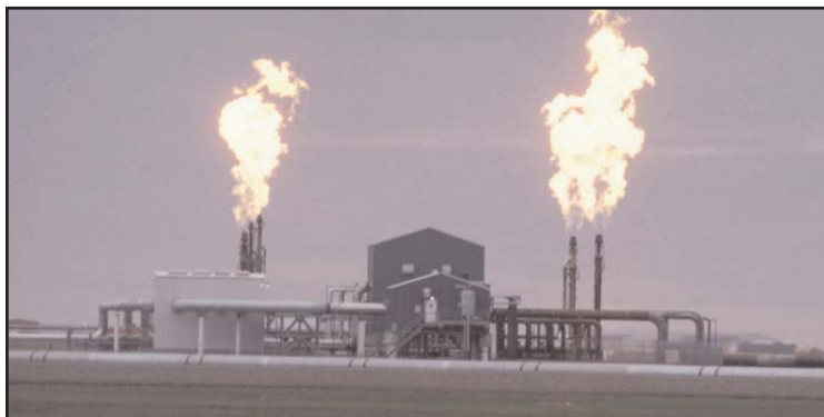
Gas flaring at Prudhoe Bay production site / Courtesy of Pamela A. Miller
